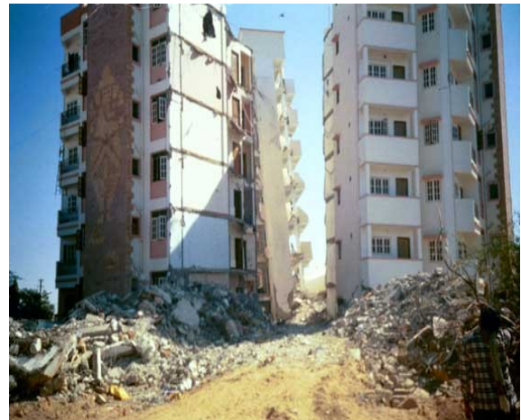
Buildings with irregular shape suffered an extensive damage in Bhuj (2001)
