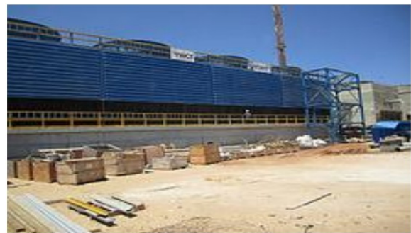
Fig: Field erected cooling tower
