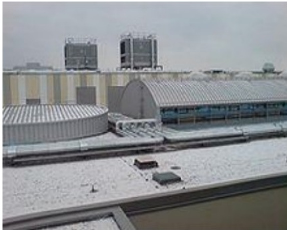
Fig: Two HVAC cooling towers on the rooftop of a shopping center (Germany)
