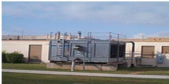
Fig: Mechanical draft cross flow cooling tower used in an HVAC application
