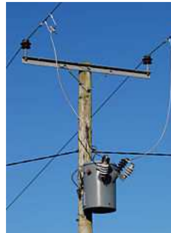
Figure 1. Phase-to-phase transformer in Britain
