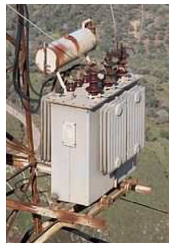
Figure 2. Three Phase distribution transformer in Syria.
