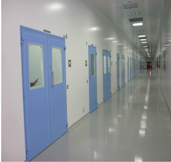
Figure 14.0 showing the frameless doors (single & Double Shutter)
