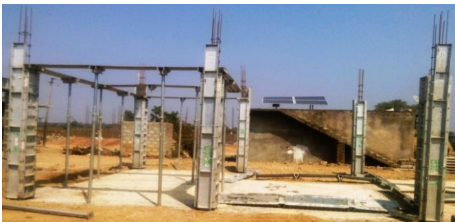
Figure 2. image of special type of form work used for construction made of aluminum.
