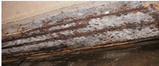
Fire damaged slab
