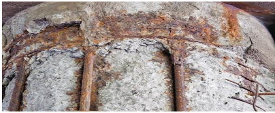
Fire damaged structure
