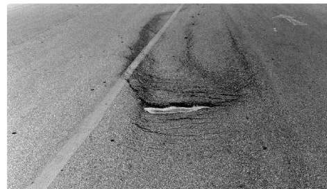
Figure 1.1: Slippage Crack ( http://www.surface-engineering.net )
