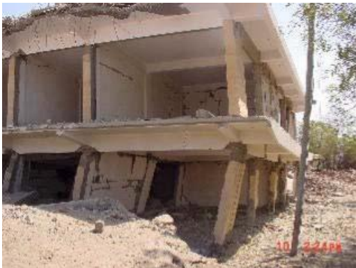
Fig. 1.4 Beam-Column joint failures
