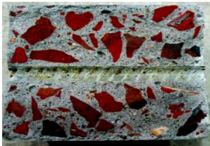
Figure 6. Broken epoxy paint coating from the pulled out steel bars.
