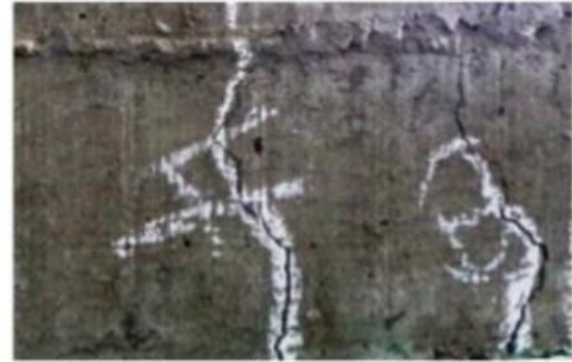
Fig -8: crack pattern and propagation in beam T-2
