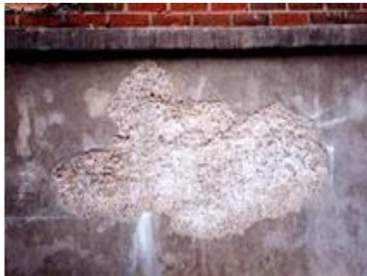
Fig 1.1 Spalling of wal
