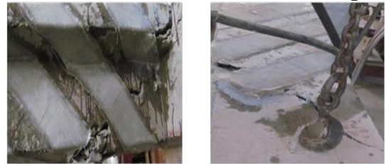
Fig.4.7 (b) Closed view of cracks Fig.4.7 (c) crack in the flange
