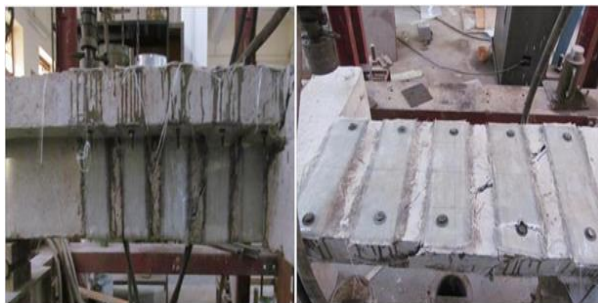
Fig 4.5(a) Closed view of Cracks
