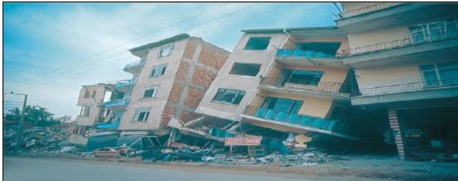
Sway mechanisms are often inevitable with soft storey ground floors (Izmit, Turkey 1999)
