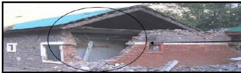
Stage III of Earthquake. Damage
