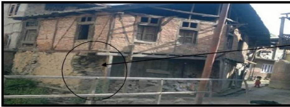
Stage III of Earthquake. Damage
