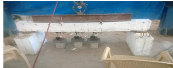
Fig-3.6 CNBM Beam Crackings.
