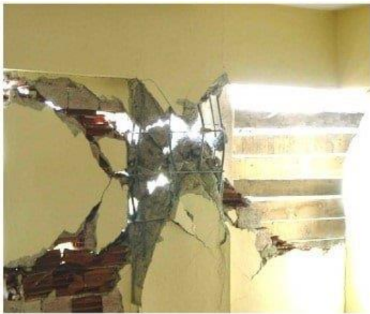
Fig:23: Brittle Failure Of Columns Asymmetric Arrangement Of Stiffness Element In The Plan:
