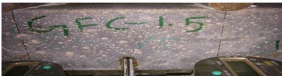
Fig. 4.6.3 Crack Pattern of GFC-1.5
