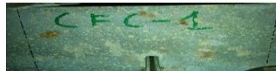
Fig. 4.6.13 Crack Pattern of CFC-1
