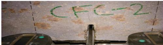
Fig. 4.6.15 Crack Pattern of CFC-2
