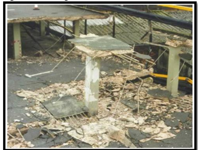
Fig: 4.2 Global collapse of the structure due to punching shear
