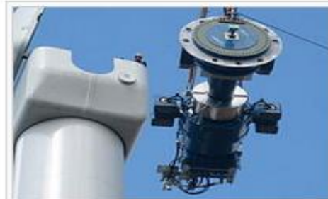
Typical components of a wind turbine (gearbox, rotor shaft and brake assembly) being lifted into position
