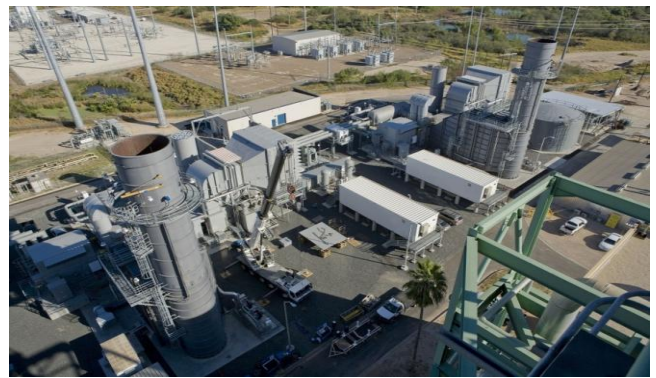
Fig : 100MW simple cycle gas turbine plant
