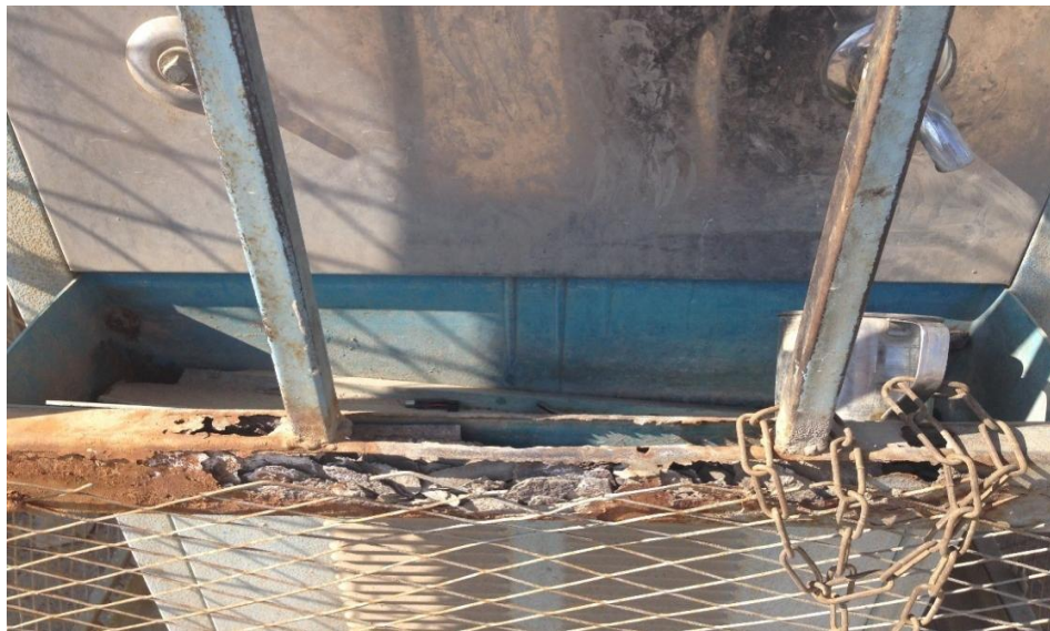
Fig. (4.). Highly contaminated water cooler, with much rust.
