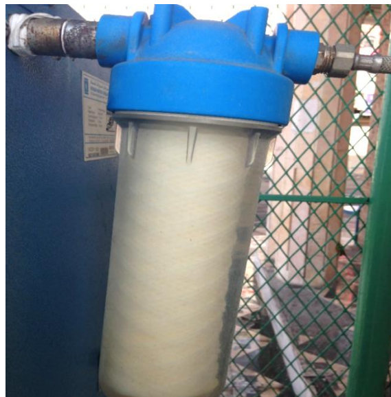
Fig. (6). A powerful filter of a newly operated cooler (one month after setting).
