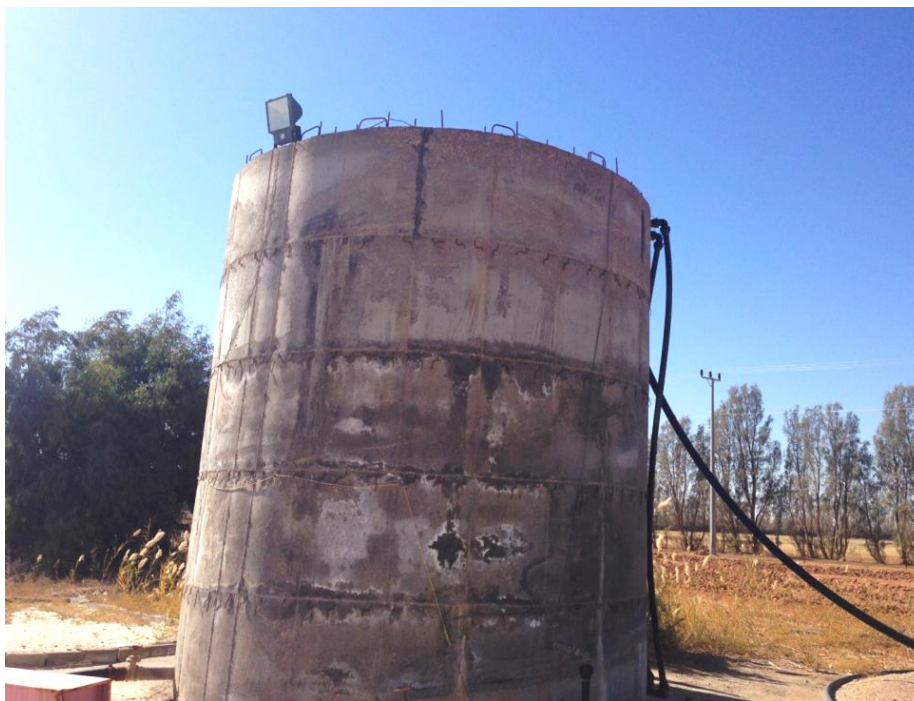
Fig. (2). A large temporary storage concrete reservoir assisting a ground water well in AlQurayyat.
