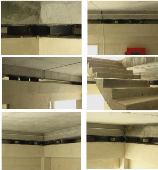
Fig. 5. Examples on installation of rubber bearings' clusters in the 17-story base isolated apartment building "Sevak" in the course of construction
