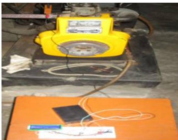
Figure 7. Temperature Sensor Set in the Air-Cooled Diesel Engine
