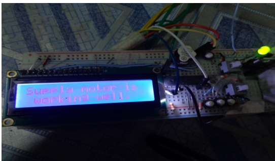
Figure 10. starting of pump with Indication of water level and motor pump condition
