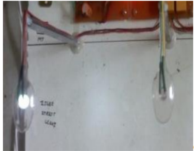
Faulty light detection (One is ON, another is OFF)
