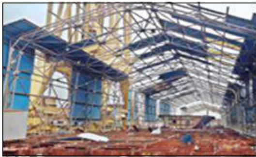
Fig.2.2 Complete damage to Hindustan Ship Yard subjected to Hud-Hud super cyclone
