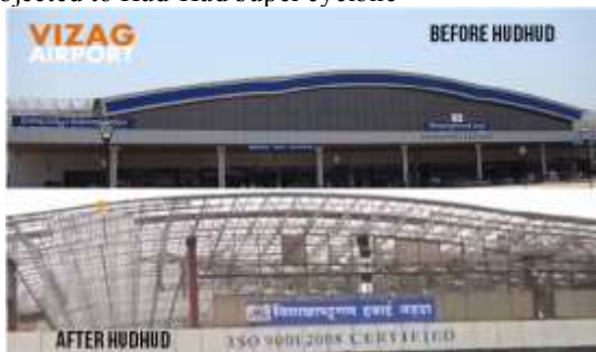
Fig.2.3 Photo showing damages to roof truss at Vizag Air Port subjected to Hud-Hud cyclone
