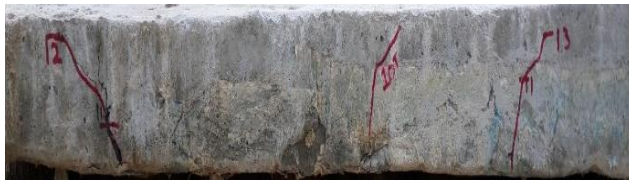
Fig. 5.8 Modes of cracks for S1 at failure
