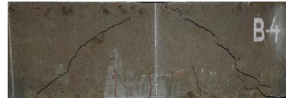
Fig. 5.7 Modes of cracks for B4 at failure
