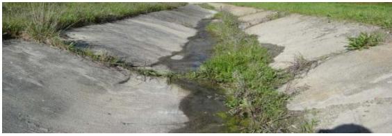
Figure.4 Concrete Lined Channel with Excessive Weed Growth
