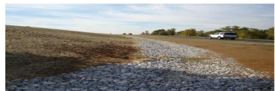
Figure 5 Small-Rock Lined Channel Outside of Clear Recovery Zone
